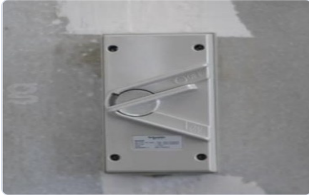
The wall switch in the OFF position.
