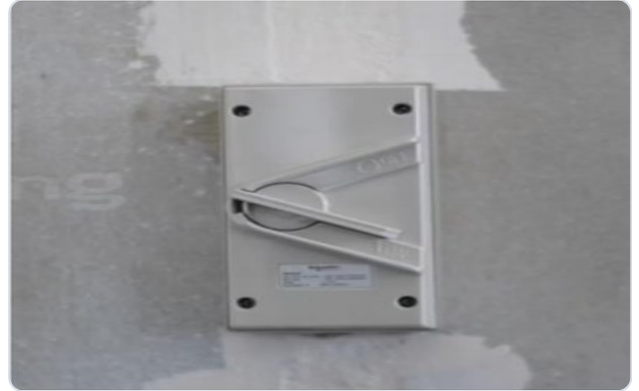
The wall switch in the ON position.
